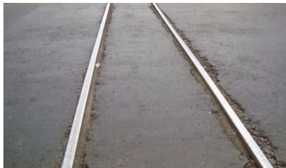
Gambar 2.14 Rusak Perpotongan Rel ( Railroad Crossing )
