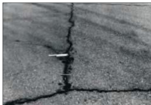
Gambar 2.8 Retak Sambung ( Joint Reflec Cracking )
