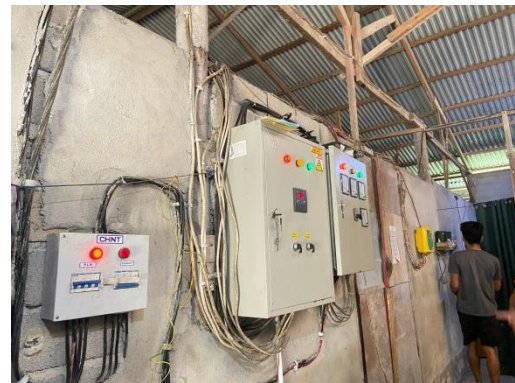
Panel- panel listrik
