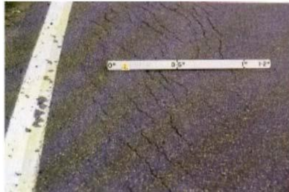
Gambar 2.17 Patah Slip ( Slippage Cracking )
