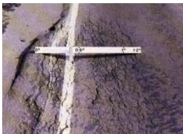
Gambar 2.16 Sungkur ( Shoving ) Sumber : Bina marga no.03/MN/B/1983
