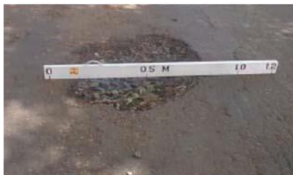
Gambar 2.13 Lubang ( Pothole ) Sumber : Bina marga no.03/MN/B/1983
