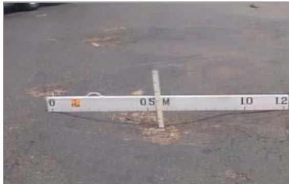
Gambar 2.6 Amblas (Depression) Sumber : Bina marga no.03/MN/B/1983
