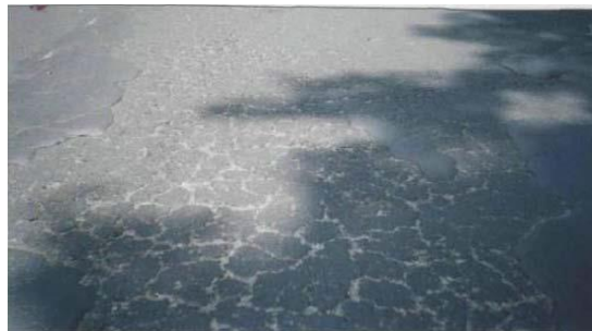
Gambar 2.19 Pelepasan Butir ( Weathering/Raveling ) Sumber : Bina marga no.03/MN/B/1983
