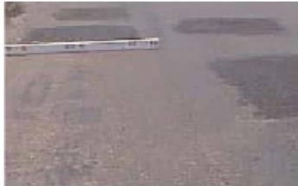
Gambar 2.11 Tambalan (Patching end Utiliti Cut Patching) Sumber : Bina marga no.03/MN/B/1983
