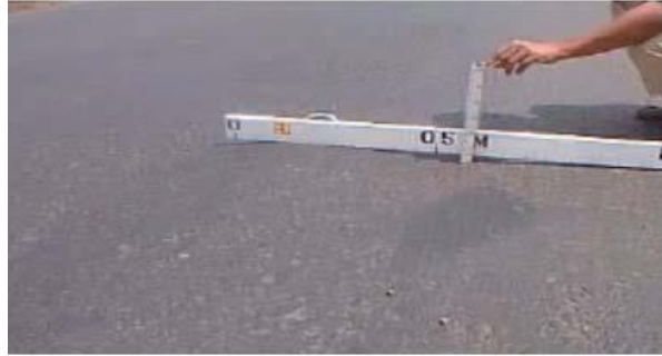
Gambar 2.15 Alur (Rutting) Sumber : Bina marga no.03/MN/B/1983
